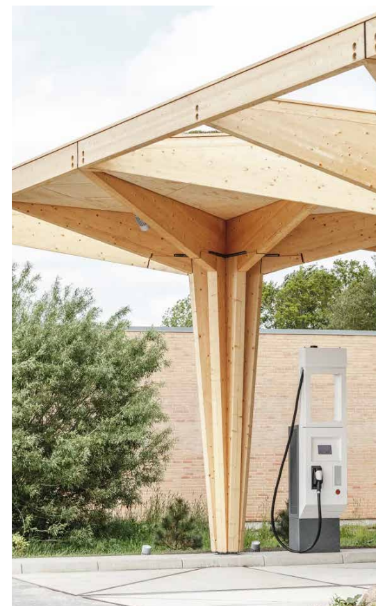
Figure 39. EV charging station at Lord's Hut Reserve and Tallangatta Showgrounds.
