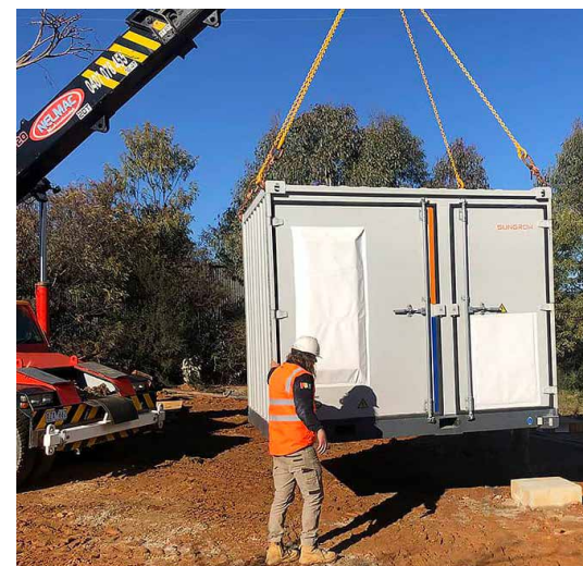
Figure 46. Modular alternate power sources. Yackandandah Town Battery.
