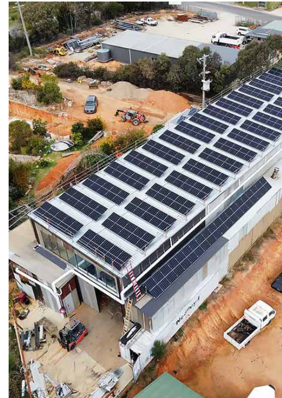
Figure 52. Alternative power sources. Yackandandah town battery.
