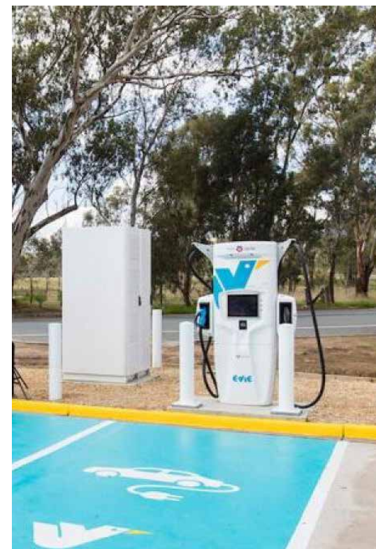
Figure 50. Electric vehicle (EV) charging station, Shepparton.
