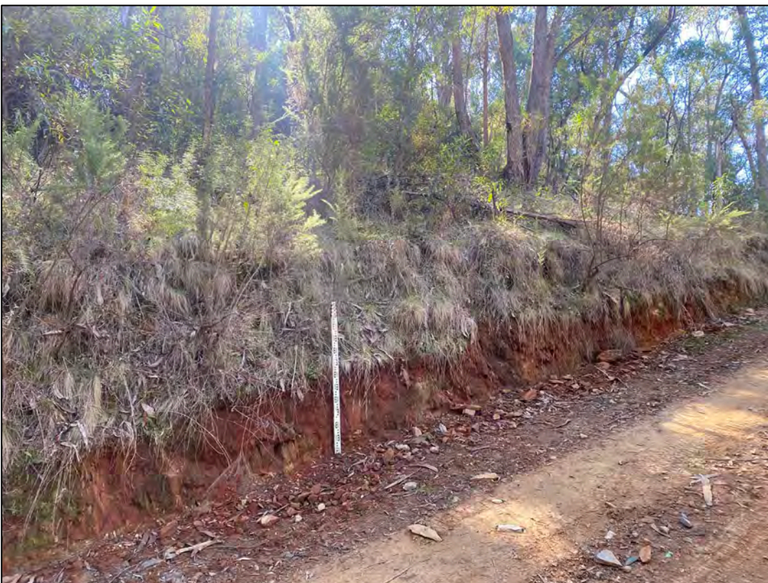
Photo 7: Midslope existing vehicle track cut-away. Poor GSV. Photo: D.Wall 2024.
